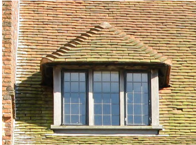
Plate 26 Hip tiles on the roof of Layer Marney Tower, Essex, which was built c. 1520
