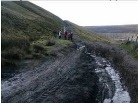
Photo: Before DCC repairs
